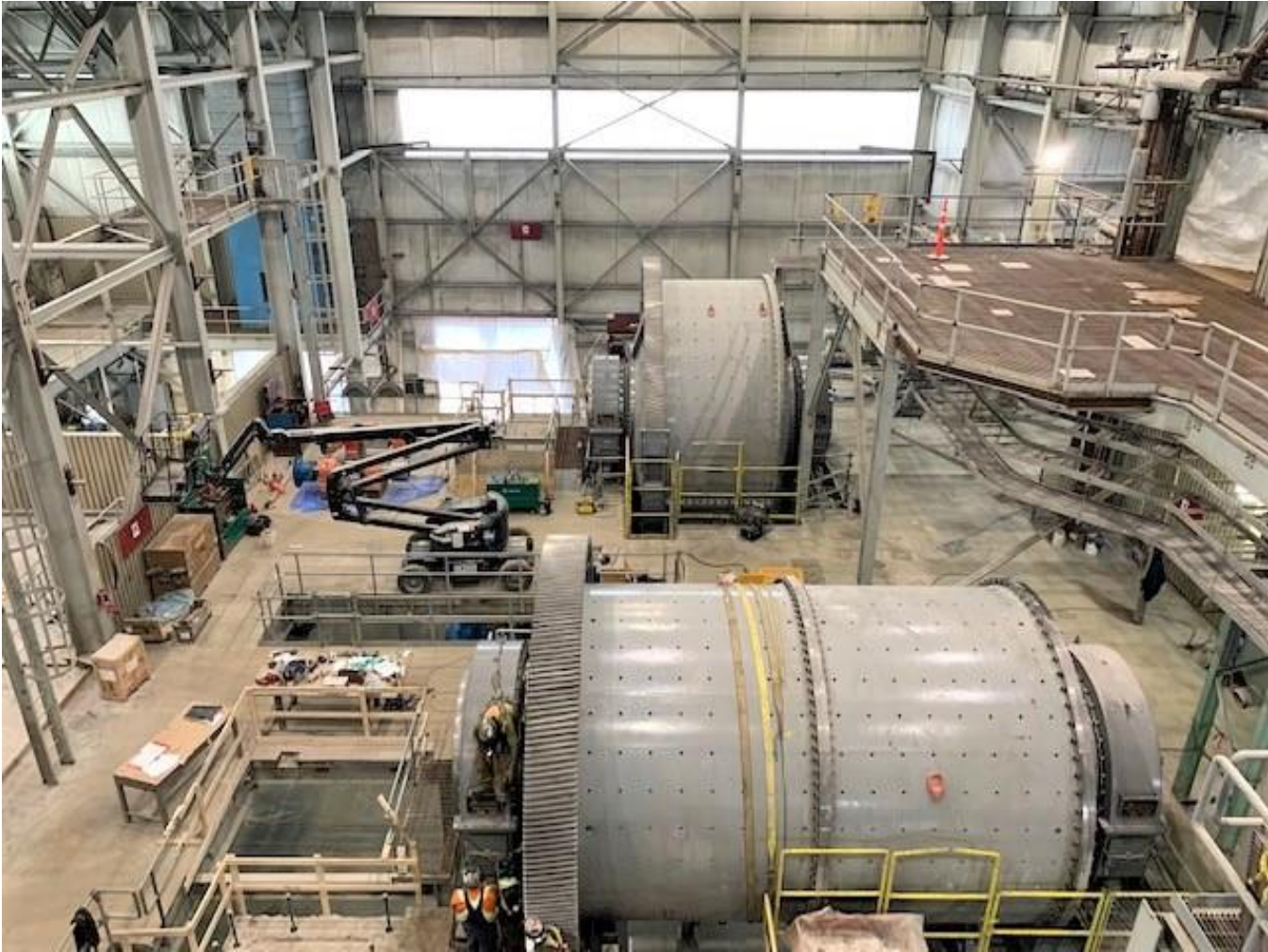
Figure 2 – Bull gears installed on SAG and Ball mills
